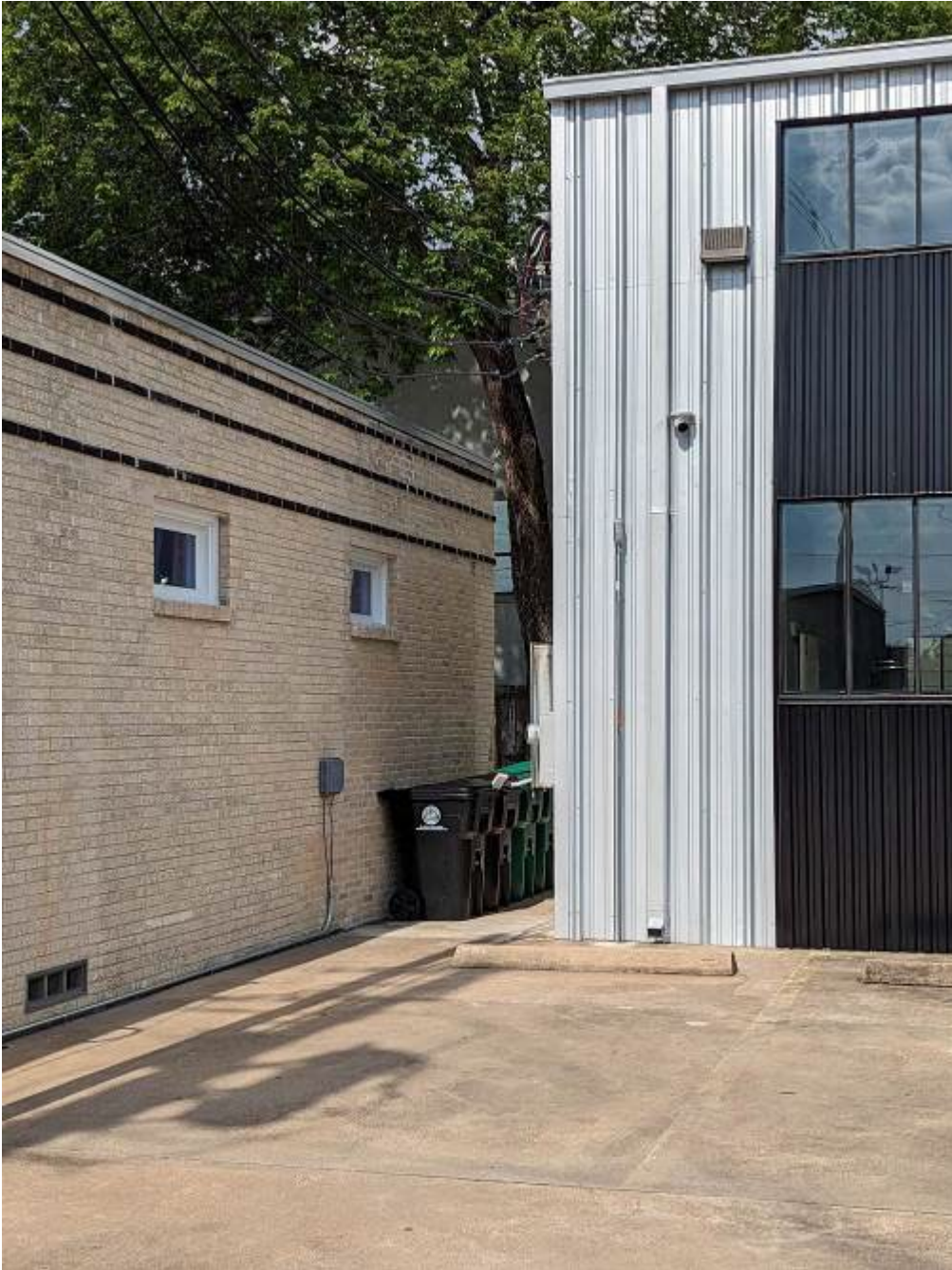
Photo 8: South Façade View Looking East at location of previous connection to adjacent metal building. 8 June 2023.
