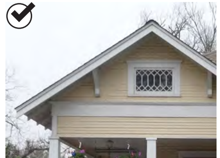
Maintain traditional overhangs: These contribute to the perception of the building's historic scale and its character.
