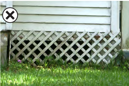
Examples of inappropriate unframed lattice
