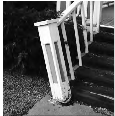
Before: A deteriorated handrail
