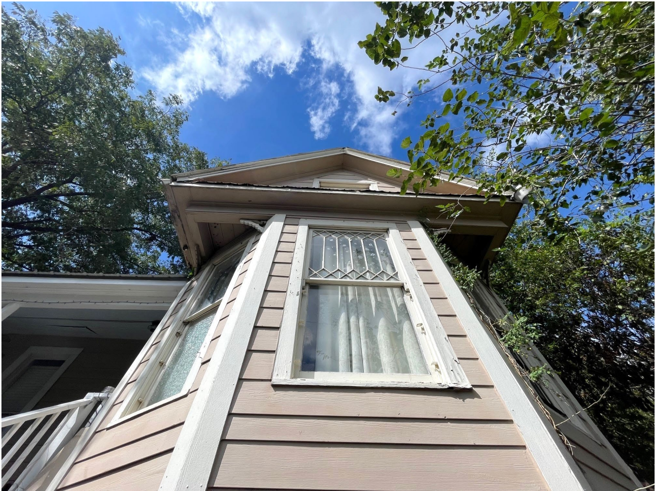
Photo 6: Original Queen Anne window detail on the primary east elevation. Photo by HOP staff member, Cara Quigley, October 6, 2023.
